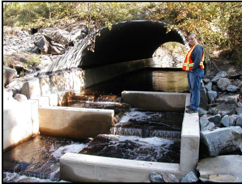
Photo 7. External Pool-and-Chute Fishway, Rt. 178 over Marsh Stream to provide adequate depth and low water velocities. Eddington, Maine. Target Species: Atlantic salmon, brook trout, and other resident species
