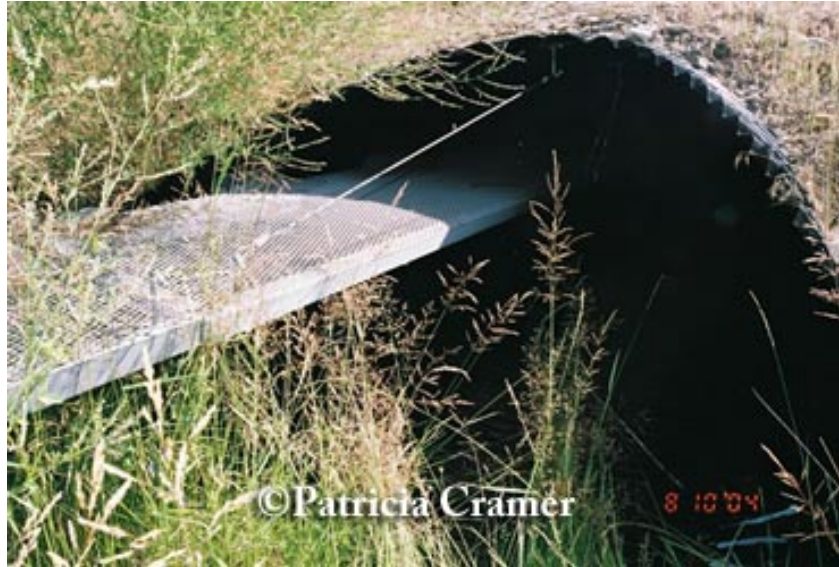
Figure 13. Small mammal shelf installed in culvert that passes water under US 93. Montana.
