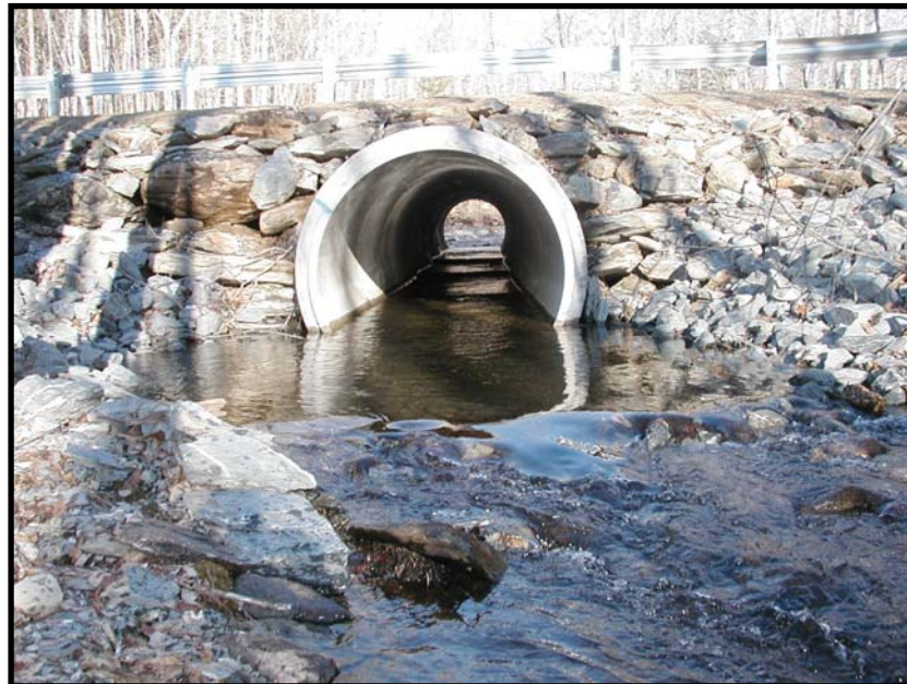
Photo 4. Reinforced Concrete Pipe (RCP) with Internal Weirs to provide adequate depth and low water velocities. Kennebec Road, Newburgh, Maine. Target Species: brook trout
