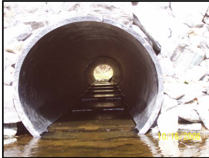
Photo 3. Slipline with Internal Weirs, Route 1 over Unnamed Stream to provide adequate depth and low water velocities. Belfast, Maine. Target Species: brook trout.
