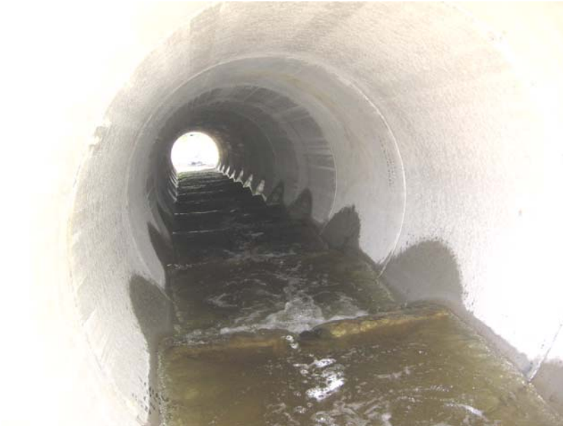
Photo 5. 8-foot Diameter Reinforced Concrete Pipe (RCP) with Precast Internal Weirs to provide adequate depth and low water velocities. Acton, Maine. Target Species: brook trout
