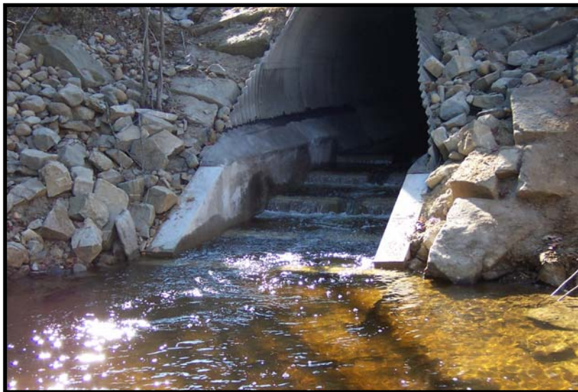
Photo 6. External Fish Ladder (with associated weirs installed during invert lining process) to provide adequate depth and low water velocities. Mill Brook, Westbrook, Maine. Target Species: alewives
