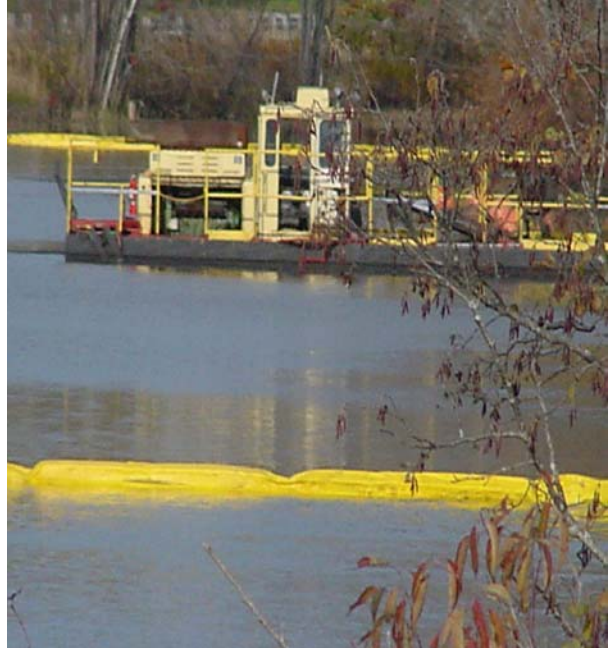
Figure 43. The dredging barge used to remove sediment and pump it to the processing location.
