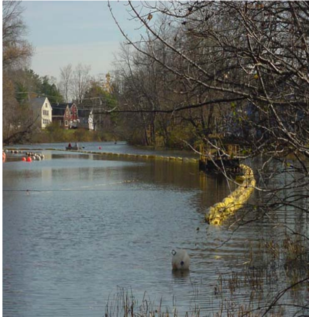
Figure 42. The silk curtain deployed around the work site to contain dredged materials.
